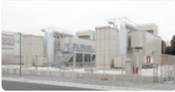
Electricity: Emergency generators
