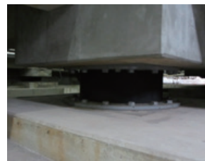
Black section below pillar shows the laminated base-isolating rubber
